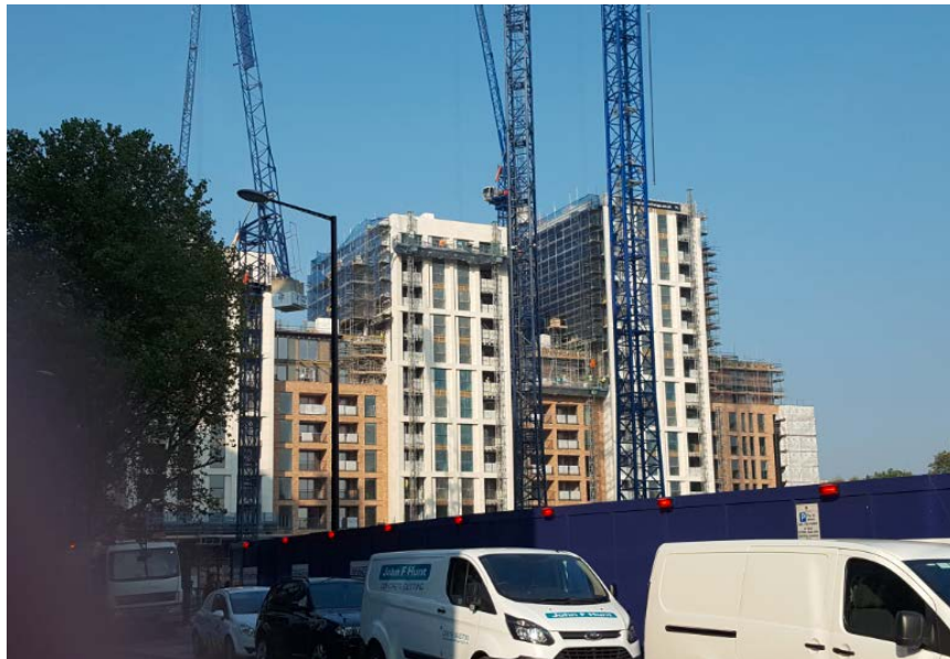
Hermitage Street (front) elevation (top) and rear elevation seen from North Wharf Road (bottom).
